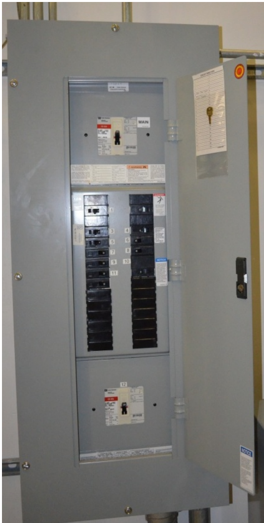
Figure 2.7 Circuit Breaker Panel
