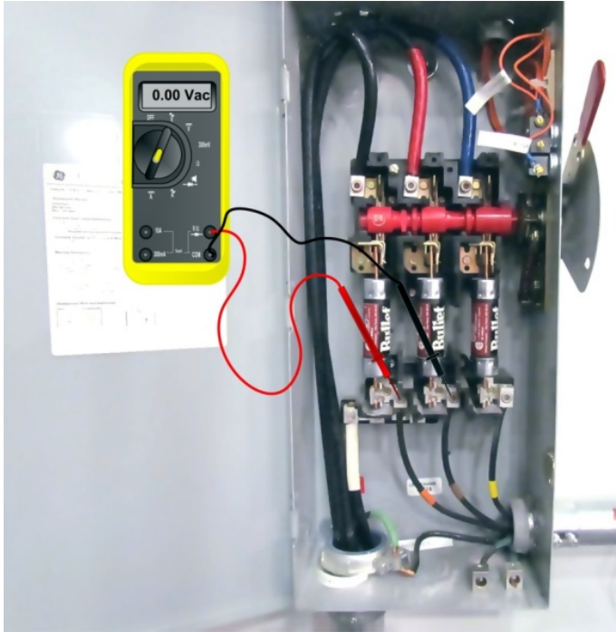
Figure 1.13 DMM Testing for Voltage Phase to Phase
