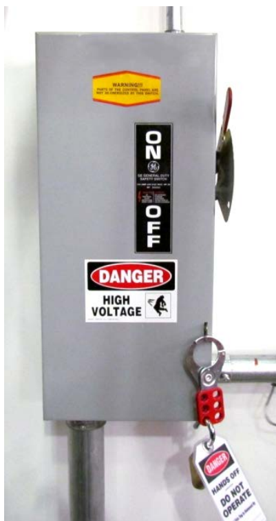
Figure 1.12 Electrical Cabinet with Lockout/Tagout Procedure Implemented
