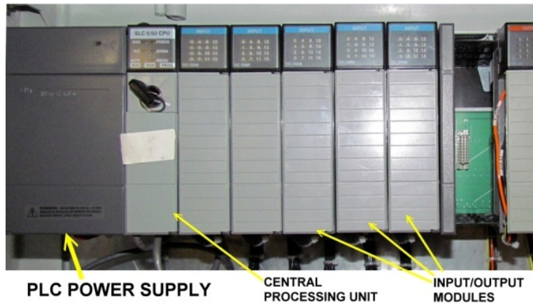
Figure 2.19 PLC Power Supply
