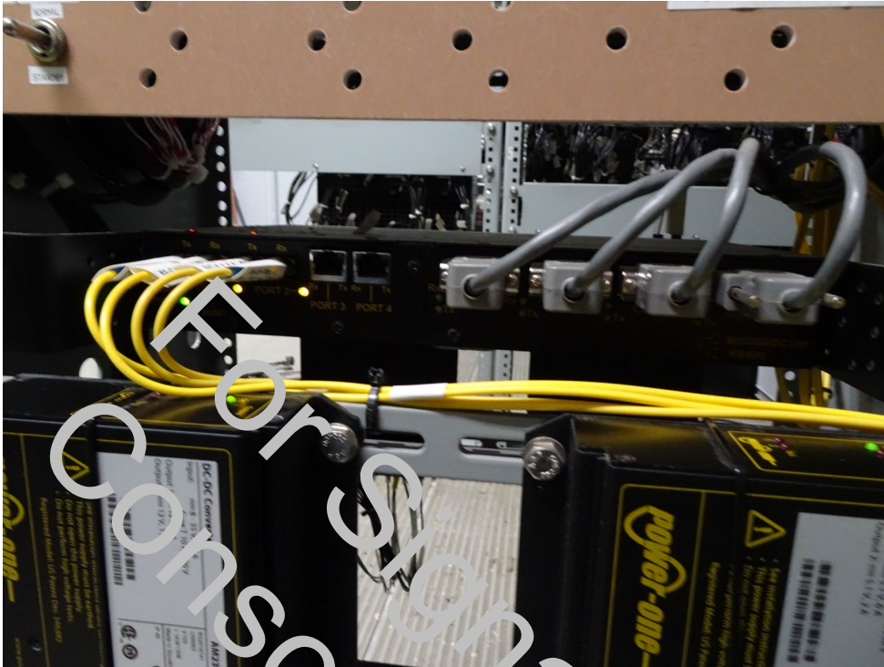
Figure 14 Modem in Transit System Operation - courtesy of SEPTA
