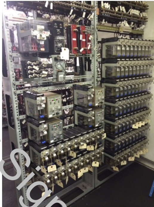
Figure 1.2 Relays in a Signal Bungalow
