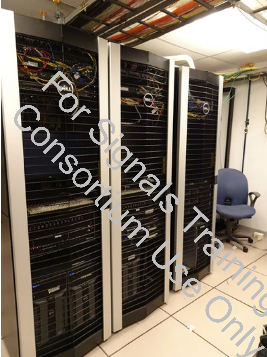
Figure 10 Part of SEPTA Mainframe Located in Central Operations - courtesy of SEPTA
